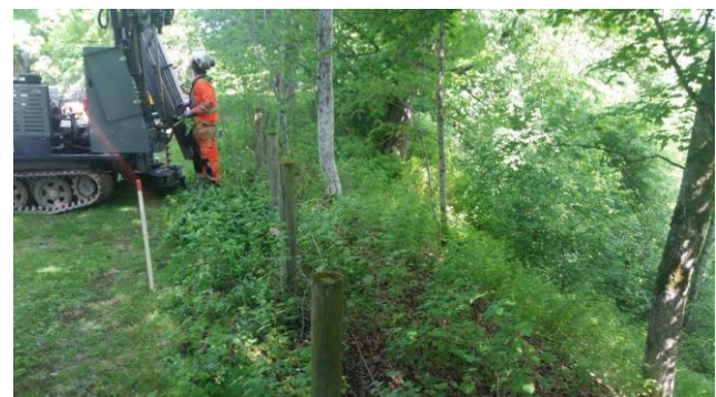
Figure 8. Installation of slope instrumentation close to the slope crest using a geotechnical drilling rig.
