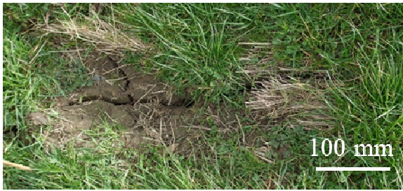
Figure 3. Typical linear cracking style on vegetated slope infrastructure in UK.
