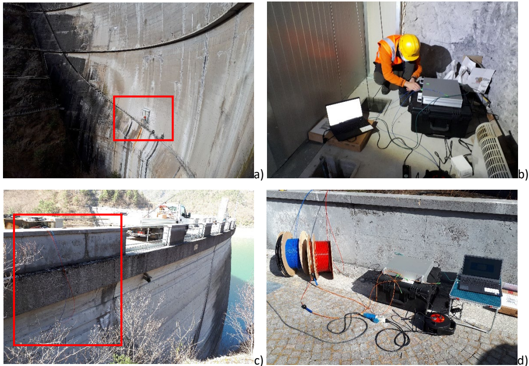
Figure 4: a) Position of the niche with respect to the dam body; b) preliminary measures in the fibers installed in the dam foundation; c) Localization of the crowning fibers; d) preliminary measures of the crowning fibers.
