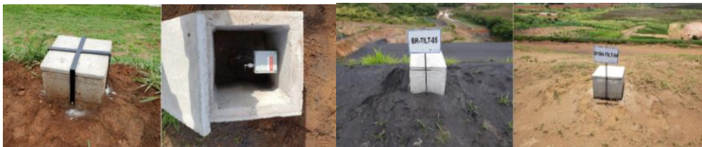
Figure 10: Tiltmeters with EDM installed by Tetra Tech in Mosaic tailings storage facilities (TSFs).
