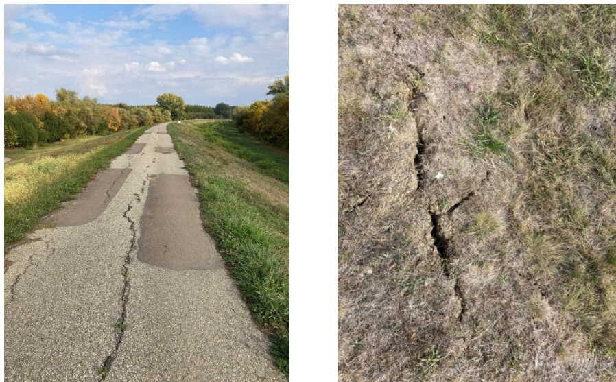
Figure 2: Paved crest of the embankment and flood side slope at Doba 87+620 tkm
