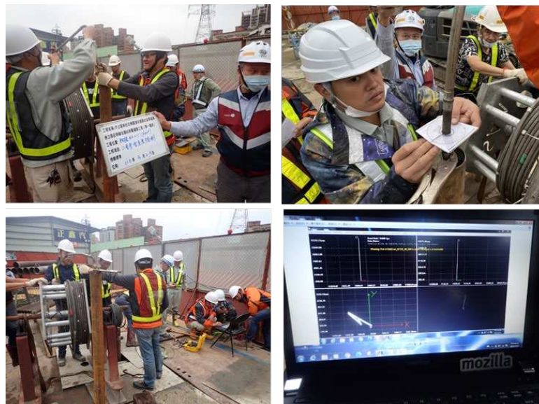
Figure 3: Photos of SAA device measurement on site.
