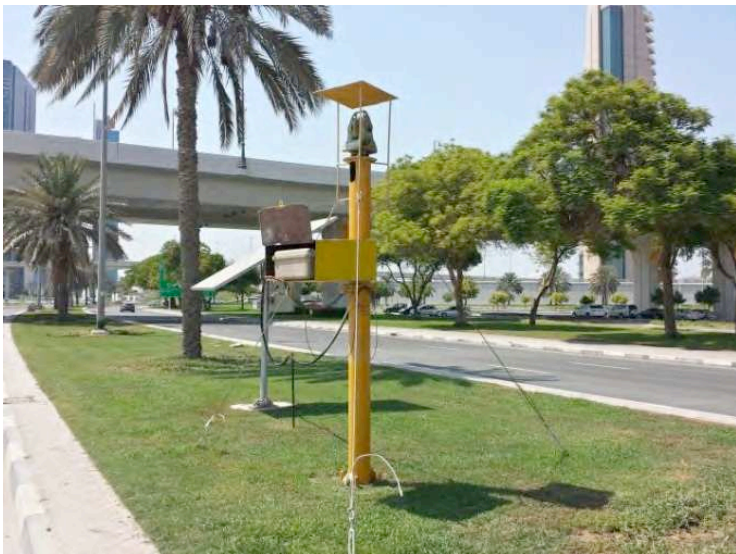
Figure 2: Installed ATS on site with control box and solar panel power supply
