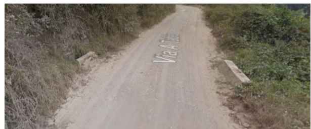
Figure 8. Drainage system of the Chía - Tabio road. Source: Adapted from (Google Maps, 2024).
