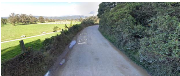
Figure 5. State of the Chía - Tabio road. Source: Adapted from (Google Maps, 2024).
