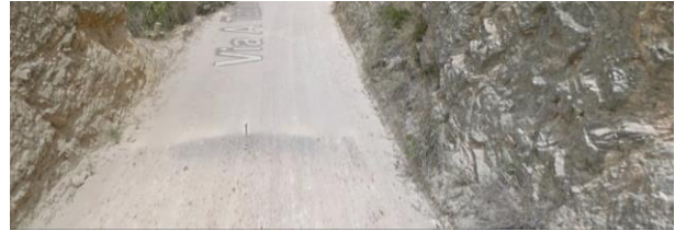
Figure 6. Unprotected rock cuts on the Chía - Tabio road. Source: Adapted from (Google Maps, 2024).
