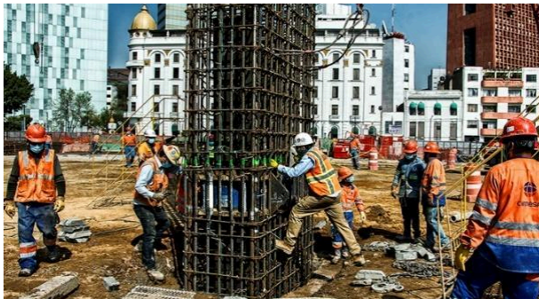
Figure 11. Reinforcement descent to drilling in the Osterberg cell area. Placement of the reinforcement cages into the drilling shaft of the test barrettes lasted up to 12 hours, because of: the instrumentation had to be installed, execution of 4 overlaps of reinforcement cages due to the 5 lifting sections and the cutting of longitudinal reinforcement at the cells zone, Figure 11.
