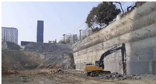
Figure 6. Shotcrete wall and active anchors in the northern area of the project.
