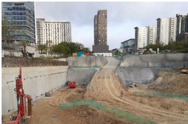
Figure 15. Southwest zone, in location of active anchors of 110 t and berm-slope for plastic screen.
