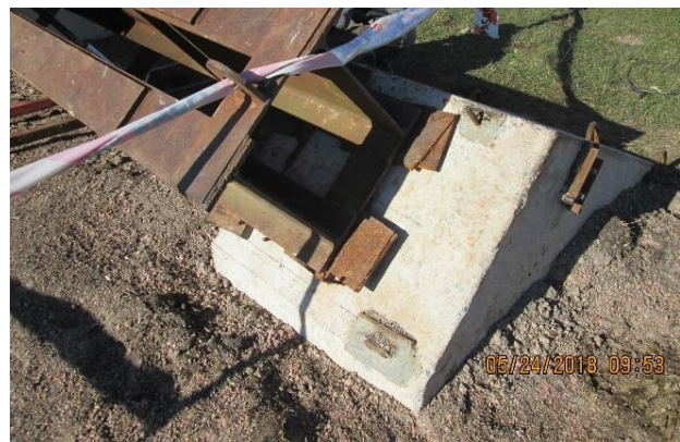
Figure 9. Failure of the reaction system support - Site 2.
