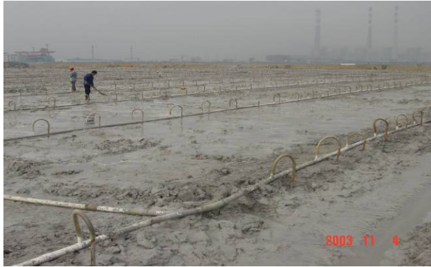
Figure 2. Array of vacuum pips and horizontal drainage pips.
