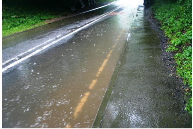
Figure 10. Flooding of the road through the defective area within the scheme
