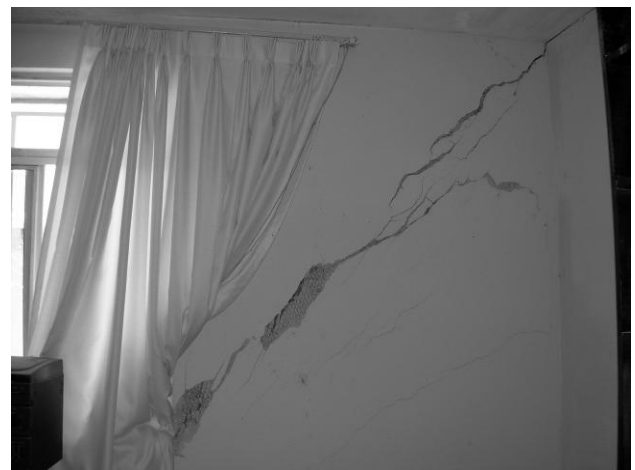
Figure 5. Diagonal cracks in a bearing wall due to diagonal tension.
