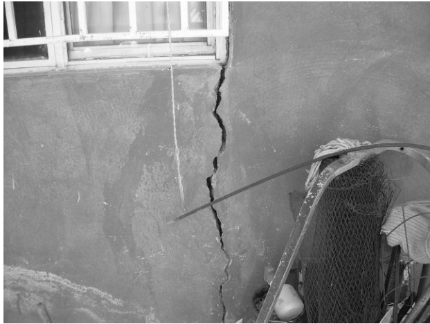
Figure 6. Vertical cracks due to differential settlement in non-reinforced walls
