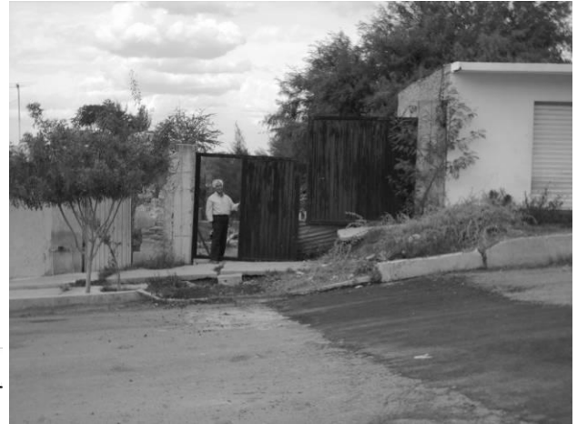
Figure 3. Ramp developed by a soil crack at the northwest of the City of Aguascalientes. The vertical displacement of the blocks generated by the rupture is evidenced by the gate.
