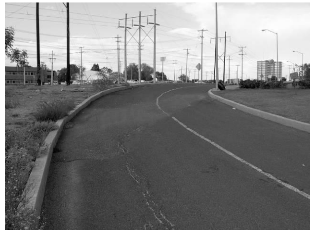
Figure 12. Cracks related to formation of caves by drag of fine material through paleochannels
