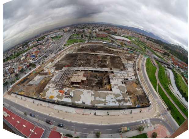
Figure 4.1 Aerial view from the east showing belt and strut slabs at first floor level.
