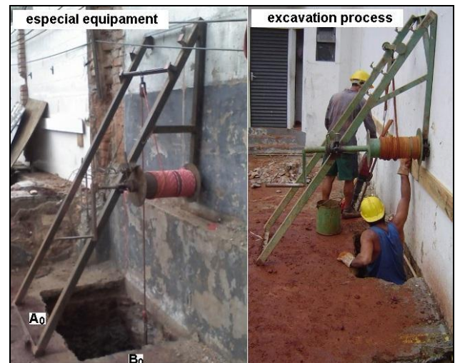
Figure 3. Special equipment and the digging process developed for big rectangular excavation within built neighborhood (Belo Horizonte, Brazil)
