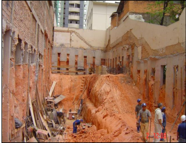
Figure 19. Intermediate stage of big rectangular in cantilever execution where it works as containment and underpinning (Belo Horizonte, Brazil).
