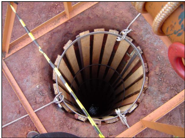
Figure 23. Use of reusable temporary shoring in a manually excavated belled caisson (Brucutu Mine, Itabira - Minas Gerais, Vale do Rio Doce Mining Company).
