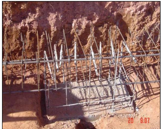
Figure 11. Big rectangular walls reinforcing steel in the distribution effort beam (Belo Horizonte, Brazil).
