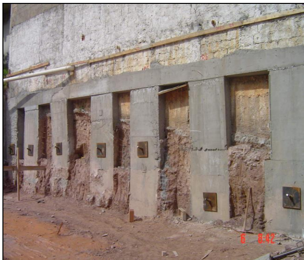
Figure 20. Intermediate stage of execution of big rectangular shored by tiebacks run in the own element (Belo Horizonte, Brazil).
