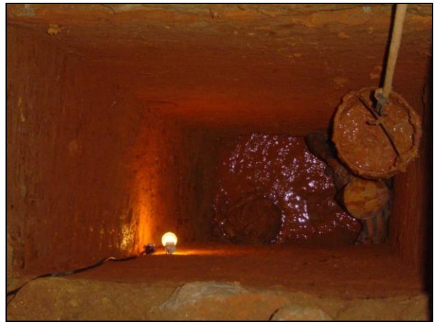
Figure 22. Big rectangular excavation in water presence with no shoring (Belo Horizonte, Brazil)
