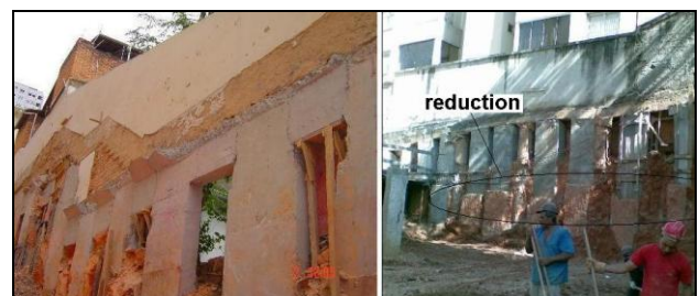
Figure 7. Examples of underpinning and retaining wall sites after front excavations and detail of a reduced section in big rectangular walls (Belo Horizonte, Brazil).
