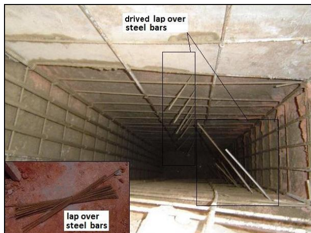
Figure 16. Lap over for supplementary curtain installed inside the big rectangular before concreting (Belo Horizonte, Brazil).
