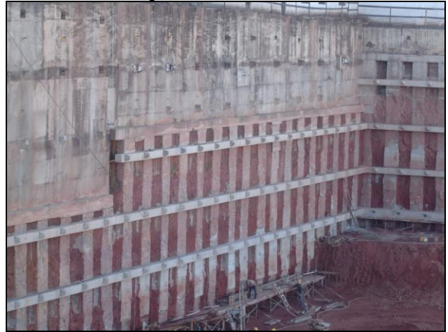
Figure 21. Intermediate stage of execution of big rectangular shored by tiebacks using distribution beams (Belo Horizonte, Brazil).
