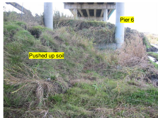
Figure 3. Soil pushed up near Pier 6 (looking south)
