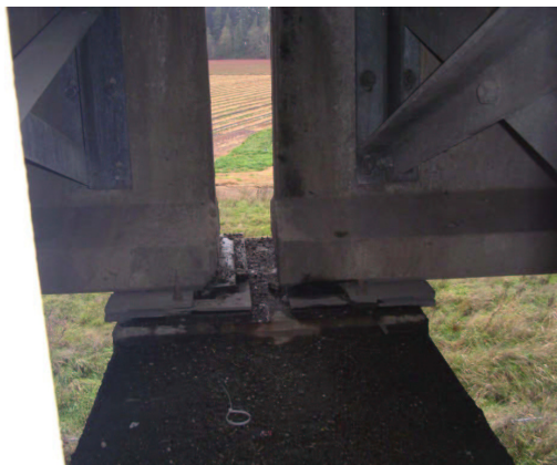
Figure 6. Displaced girder at Pier 6 (looking west)
