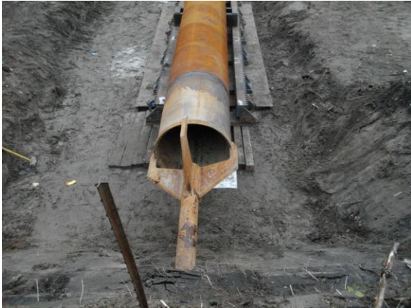
Figure 5. "Spider" attachment connecting 30 inch casing for first Installation to 6 inch pilot string, protruding from embankment.
