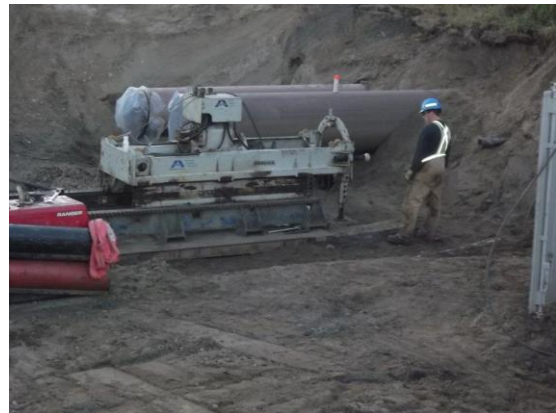
Figure 4. Bore rig preparing to install 6 inch pilot hole beside first two installed pipelines.
