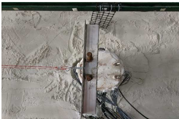
Figure 9. Cracking and gap formation in the crust post-earthquake.
