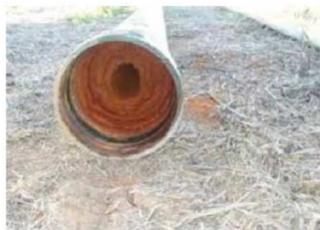
Figure 3. Duct clogging due to ochre accumulation.
