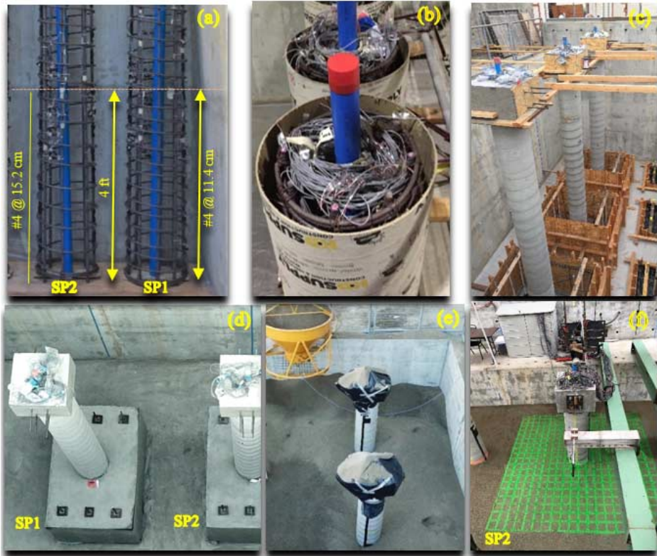
Figure 4. (a) Pile rebar cages, (b) Instrumented specimens prior to concrete pouring, (c) Concrete piles placed in rock-socket formwork, (d) Specimens with rock-sockets anchored into the floor after formwork removal (e) Sand pluviator, (f) Completed test setup for SP 2.
