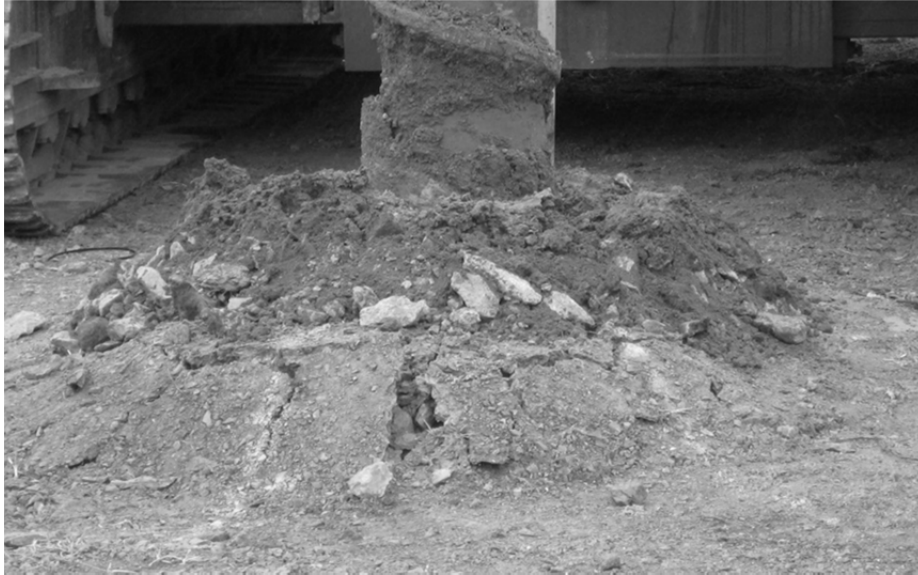
Figure 5. Ground heave occurring during the installation of test pile E (axis B-B)
