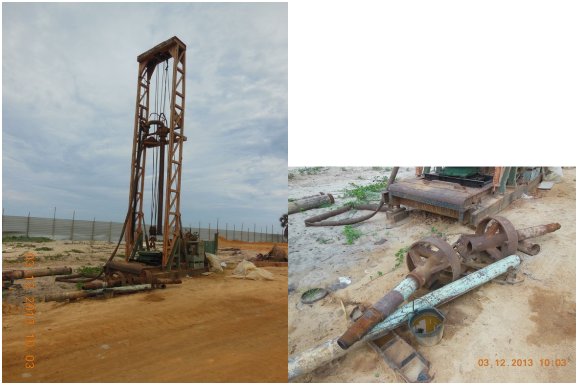
Figure 2. Piling rig (Jintai GPS-15) and drill bit used for test pile installation
