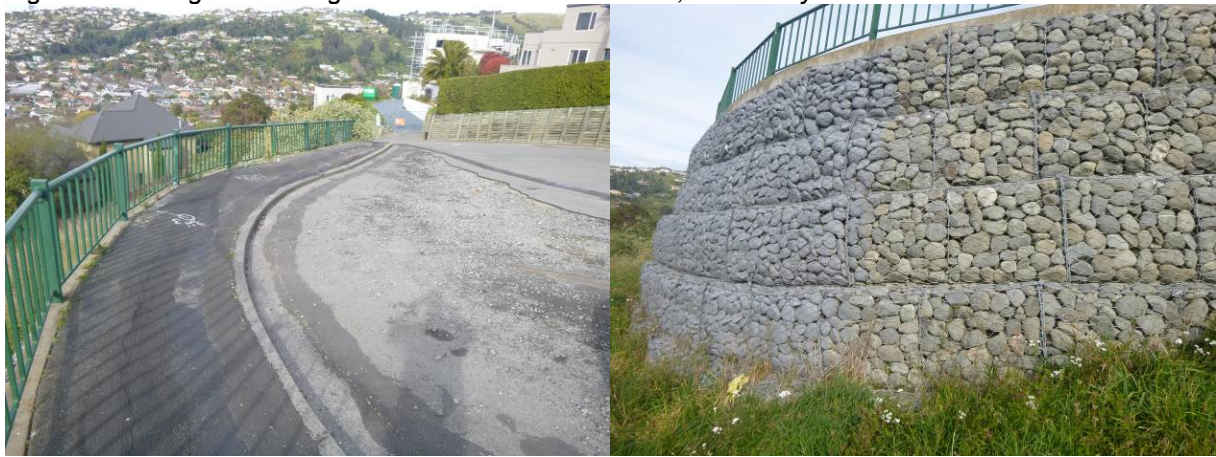
Figure 6. Damage of mesh gabion wall
