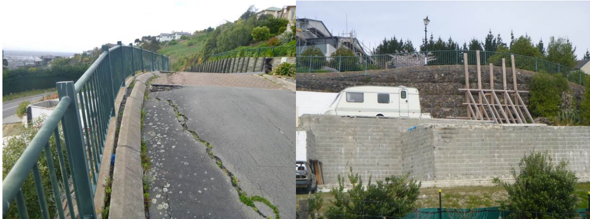
Figure 5. Damage of mesh gabion wall – Yelverton Place, Huntsbury
