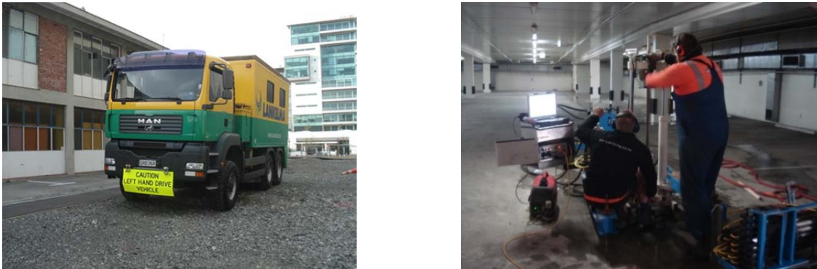
Figure 1. CPT truck (left) and portable CPT rig operating from the basement of the building (right).
