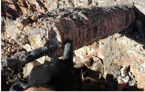
Figure 4. Ribs on the exposed grout column
