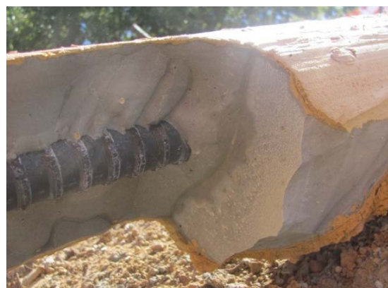
Figure 9. Soil smear on the pulled [ungrooved] grout column
