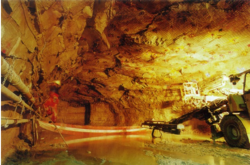
Figure 2. Storage gallery top heading excavation prior to trimming showing Hawkesbury Sandstone strata, groundwater inflow, rock bolt roof support and temporary safety mesh.
