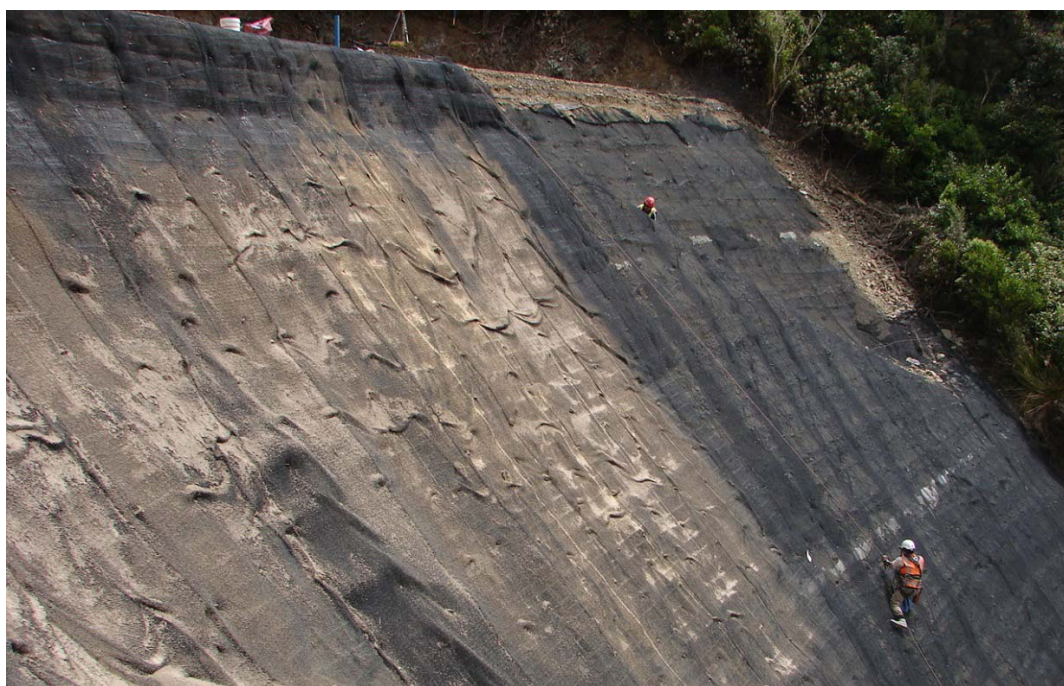
Figure 4. Installation of Erosion Protection Mat on the Face of Reinforced Soil Embankment
