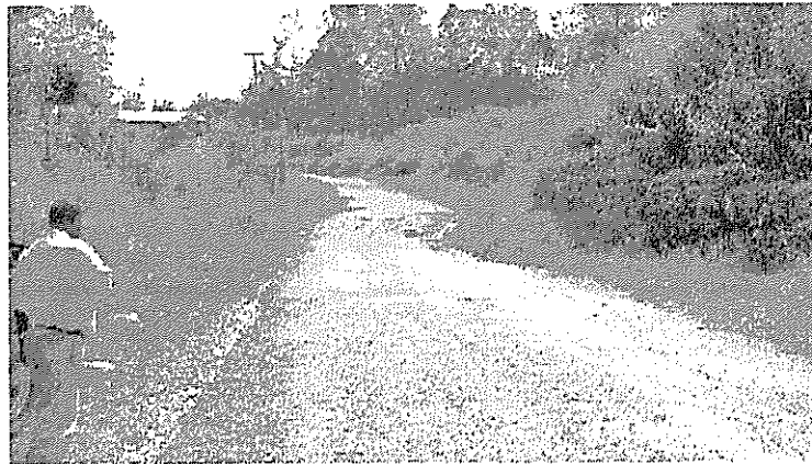
Figure 6. Overriding earthflow partly blocks the highway in eastern Simbu Province. Note also the lateral shear that displaces the road pavement.
