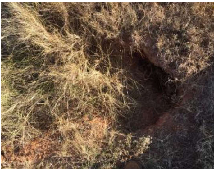
Figure 10 Observed sinkhole feature (Diameter approximately 0.4m)
