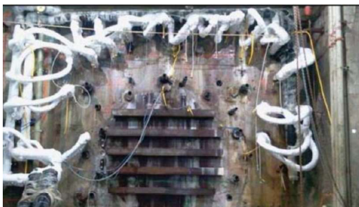
Figure 9. Freezing in COB for tunnel break-out and connection (after Polycarpe et al. 2012)
