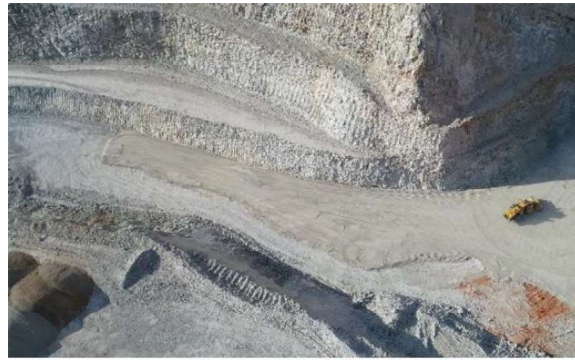
Figure 3. Aerial of the first layer of fill material being placed. Example of the aeolian sand backfill can be seen in the bottom right.
