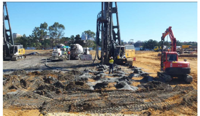
Figure 5. Concurrent activities on site, this picture shows 4 concrete trucks, 2 CMC rigs, auger rig and low loader truck.
