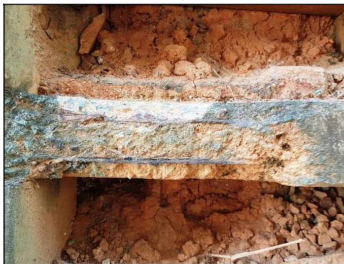
Figure 2. Corrosion induced spalling of concrete crib wall units.
