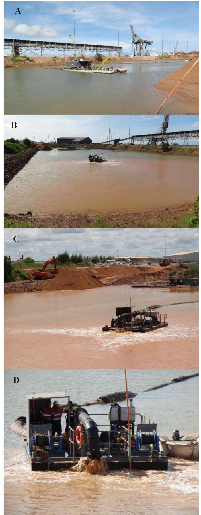
Figure 4 (A) Cutter suction dredge within the pond pumping sand to (B) a pontoon depositing material over soft soils. (C) Quarried sand was transported to site and carefully placed into the pond for dredging and transportation. (D) A closer view of the pontoon showing the diffuser spreading sand upon the soft muds
