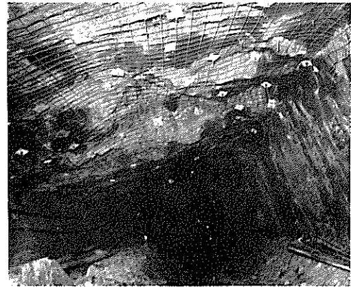
Fig. 2 Tensioned Rock Bolts and Steel Mesh installed in a Mechanized Cut and Fill Mining Operation. (Courtesy of Mount Isa Mines Limited, Australia)
