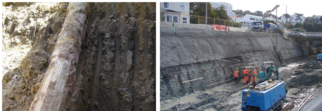
Figure 3: (a) Exhumed trial soil nail showing post-grout (pink), and (b) construction of soil nail wall
