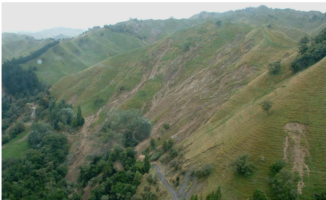
Figure 1: Aerial view of landslips Turakina Valley Road
