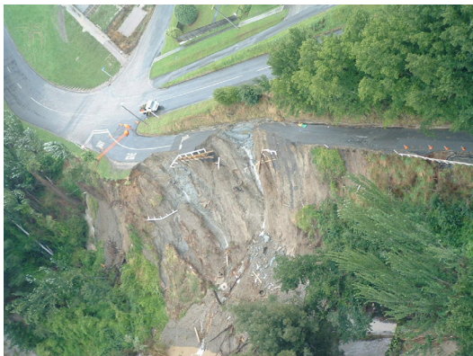
Figure 12. Papakai Road failure
