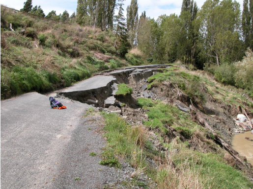
Figure 10. Otaihape Slip after failure.
