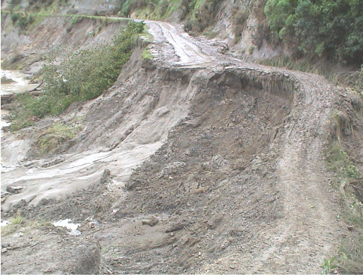
Figure 7. Failure prior to re-contouring
