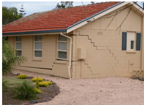
Figure 15: Example of house distorted by collapsing soil movement
