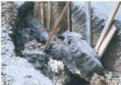
Figure 1: Instability of an excavation in expansive clay
