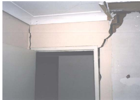
Figure 2: Expansive soil effects on domestic structure
