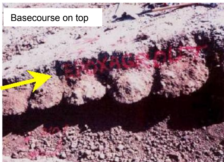
Semi-contiguous cemented bulbs (NB. Concrete removed)
