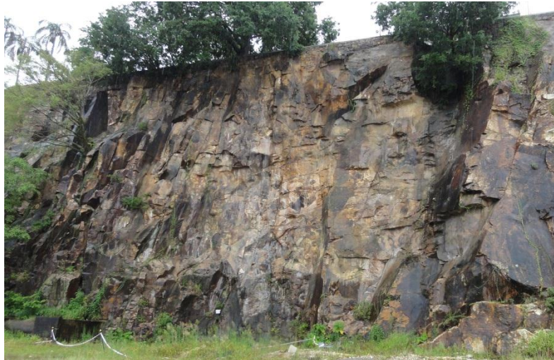
Figure 3 - Typical Tuff jointing with wedge failure at right at crest
