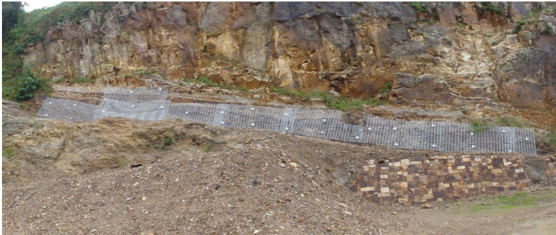
Figure 5 - Unconformity treatment after initial collapse in January 2011.
