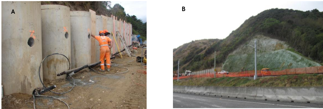
Figure 4. Exposed upper part of a 10 m high soldier pile wall with rock anchors under construction (a), widening of the railway corridor by using soldier pile walls and cut slopes (b)
