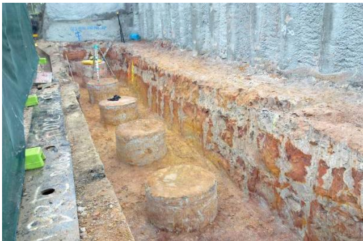
Figure 4. Exposed pile heads at Pier 1
