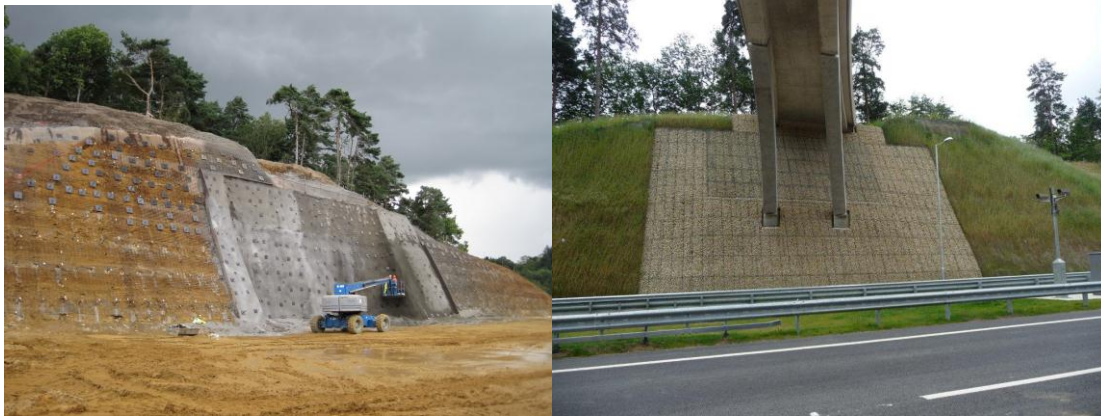
Figures 4 & 5 – Miss Jame’s Bridge 60° cutting rigid and hard facing during construction and post construction
