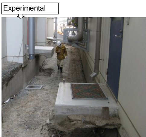
Figure 11. Ground subsidence around the building
