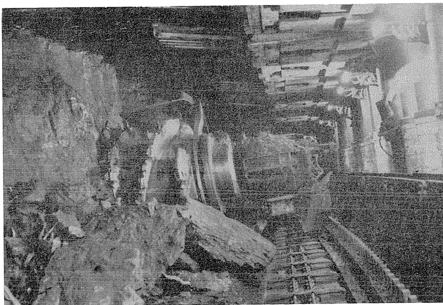
Figure 3 Longwall face installations
