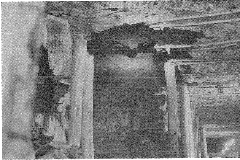
Figure 9 Conditions of roadway in B heading, 471 Panel, in sandstone area showing effect of high pressures
