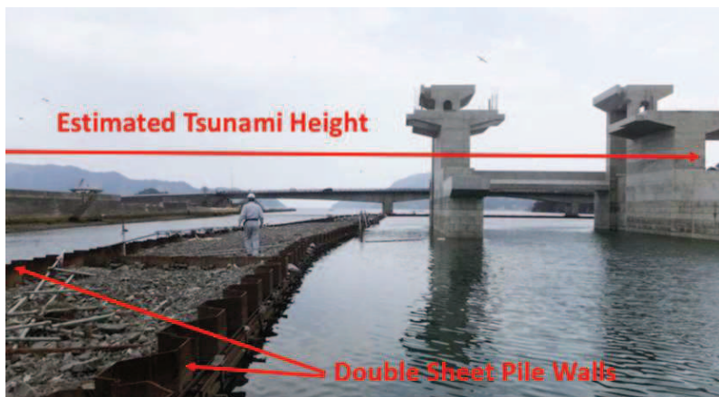
Figure 3. Almost intact double sheet pile wall cofferdam after 9m-high tsunami overtopping
