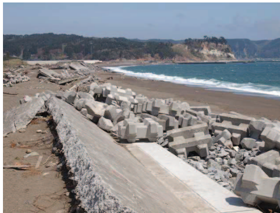
Figure 1. Heavily damaged coastal levee of Noda, Iwate Prefecture (Tohoku Regional Bureau, Japan Ministry of Land, Infrastructure, Transport and Tourism)
