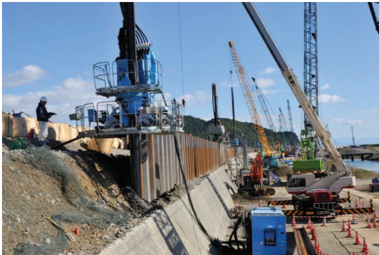
Figure 6. Press-in work of sheet piles into the existing levee at multiple sections
